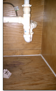
Monitor under a well-sealed sink
